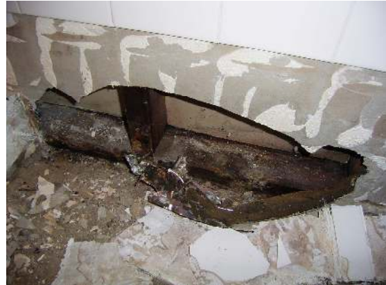
3. Repair or replace broken wall sheeting if required
